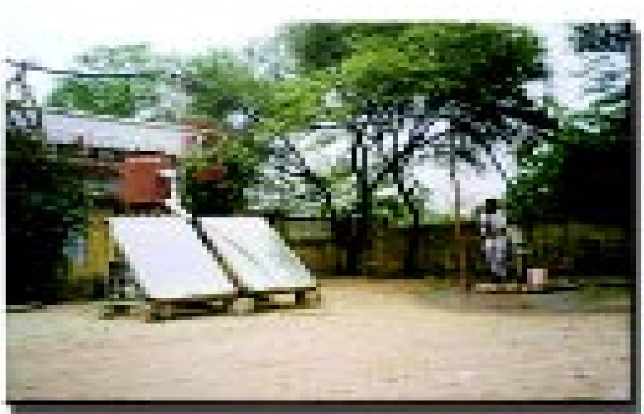
Solar power for water heating
