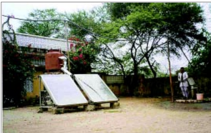
Solar power for water heating
