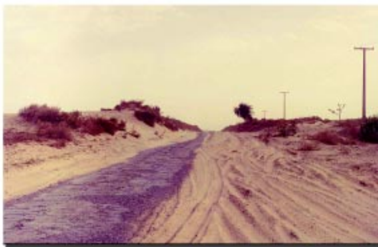
Encroachment of moving sand onto roads
