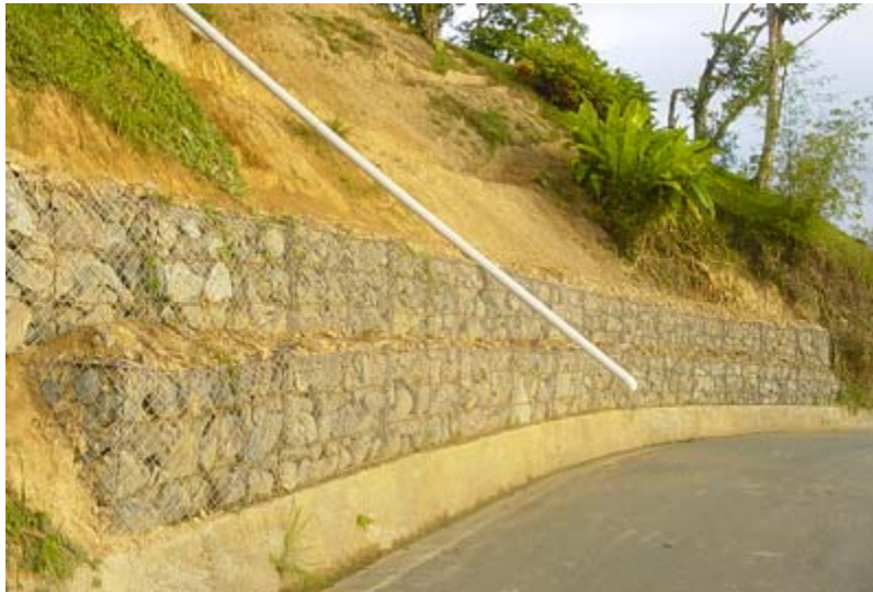
Photograph 24: Gabion baskets, a low tech method, are used to curb erosion and landslide, but still expensive to low and middle income homeowner
