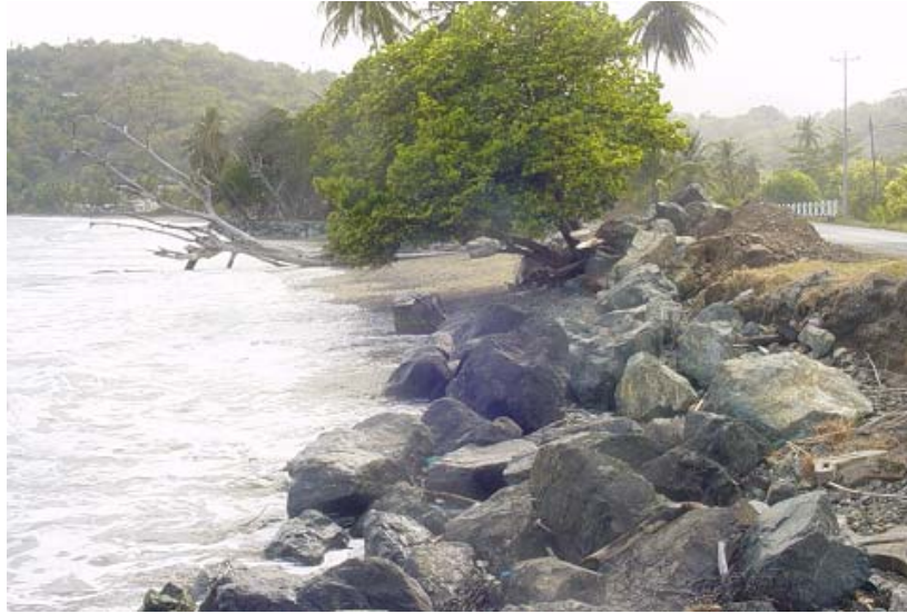
Photograph 21: Faulty Coastal Defence Works, Goldsborough, Tobago
